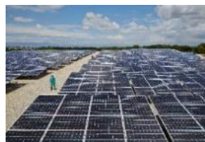
Solar power generation
