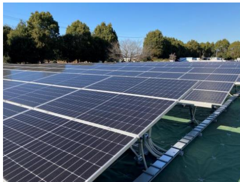
Introduced solar power generation at our MDC
