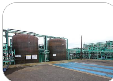
Seki Business Office (water treatment)
