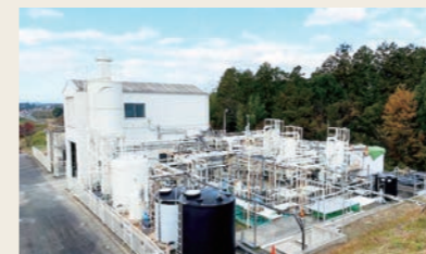
Wastewater treatment facilities at the Okayama Plant
