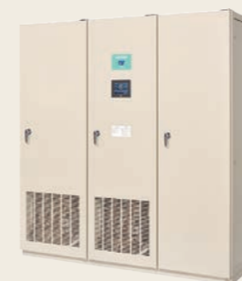
Uninterruptible power supplies (UPS)
