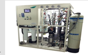
Pure water production system
