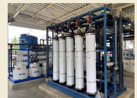
Reverse osmosis membrane filtration water purification system
