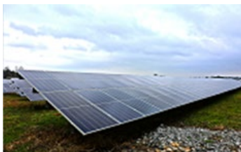
Brighter Future Solar Power Generation
