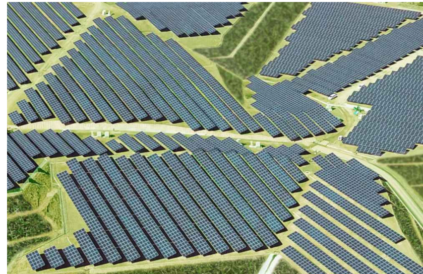
Kakuda Solar Power Plant
