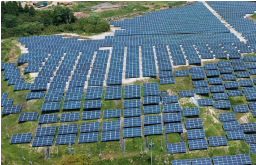
Kunisaki Solar Power Plant
