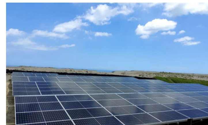
[WWB Kamisu Solar Power Plant] An example of an operational project developed in Kamisu, Ibaraki Prefecture.
