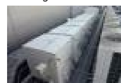
Ice storage air conditioning system
