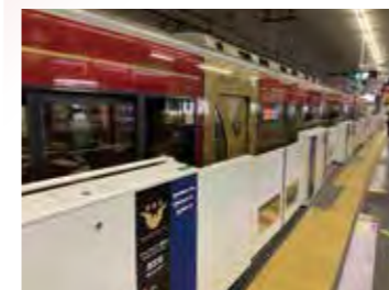
Platform screen doors will be installed on eight tracks in four stations, including Hirakata Station, by FY2026
